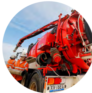
Image above: Service investigations will soon get underway across the project area.
